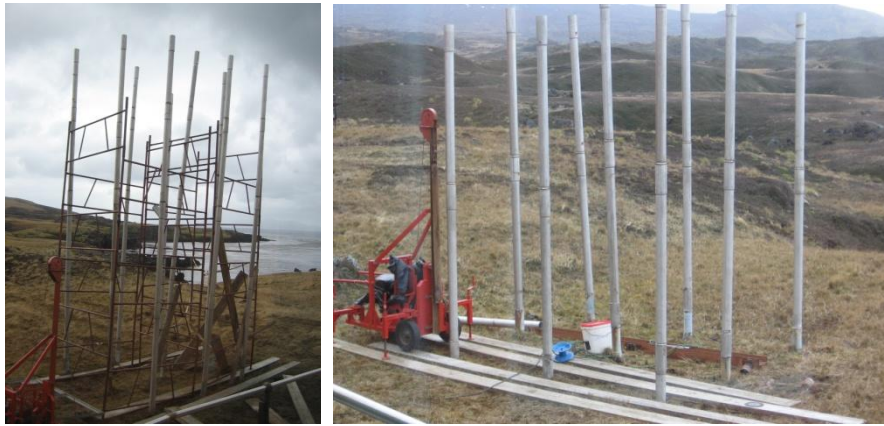
Early day of erecting the mast; the pipes are stainless steel and are hit into the earth with this red machine until they 'rest' on rock. The mast has 9 legs and stands about 15m high.
