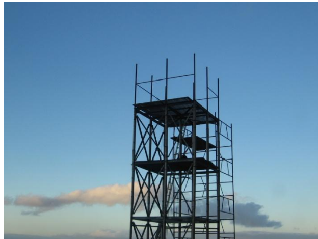
Almost completed. It will have a ladder and a cable tray all the way to the top.
